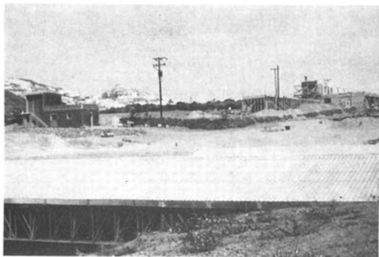
1. A view of the excavation. Lower part, the great shed B; upper left, the little Museum and staff quarter; upper right, laboratories, store-rooms and the technical personnels quarter.
