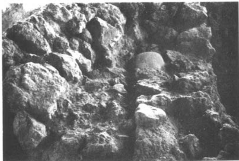
1. The broken wall of the previous pictures. The lower part (to the right) stands still upright. Left side, the fallen part. Middle section: the space between the upright and the fallen parts of the wall, full of debris.
