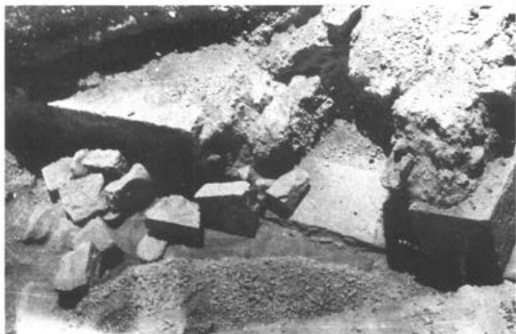
Fig. 51. Bronos 1a. The North wall of the building in ashlar masonry. The traces of the earthquake are visible.
